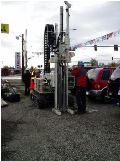
Soil gas samples outside of the building are installed with a small drill rig, using steel rods that are driven to collect the sample and then removed.
