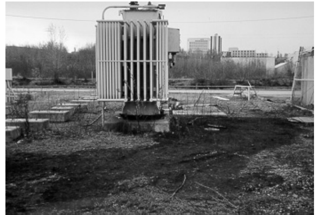
Soils stained after mineral oil containing low-level PCBs spilled from out-of-service transformers.
