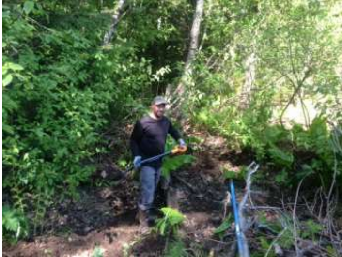
TWC Staff clearing debris from the drainage ditch flowing into the constructed wetland. Photo: TWC Staff
