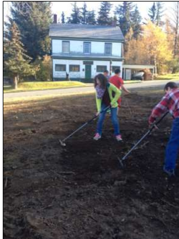
Middle School students complete the final grading at the newly constructed bioswale in the Fort Seward Parade Grounds. Photo: TWC Staff
