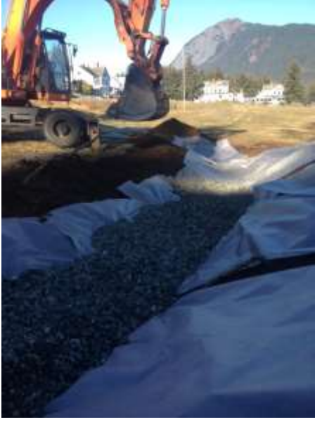
Swale lined with geotextile and filled with drain rock. Photo: TWC staff
