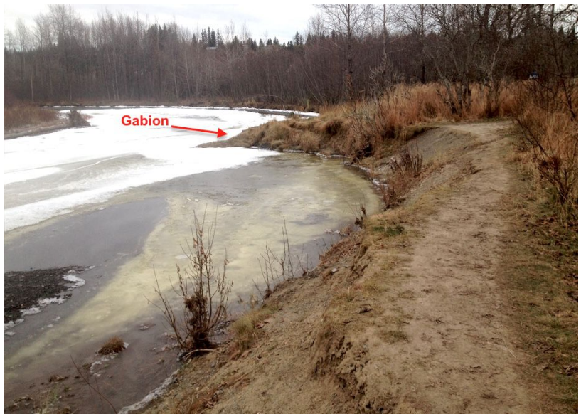
Above: Looking upstream towards gabion; bank vegetated and eroding, HSWCD 11-6-18
