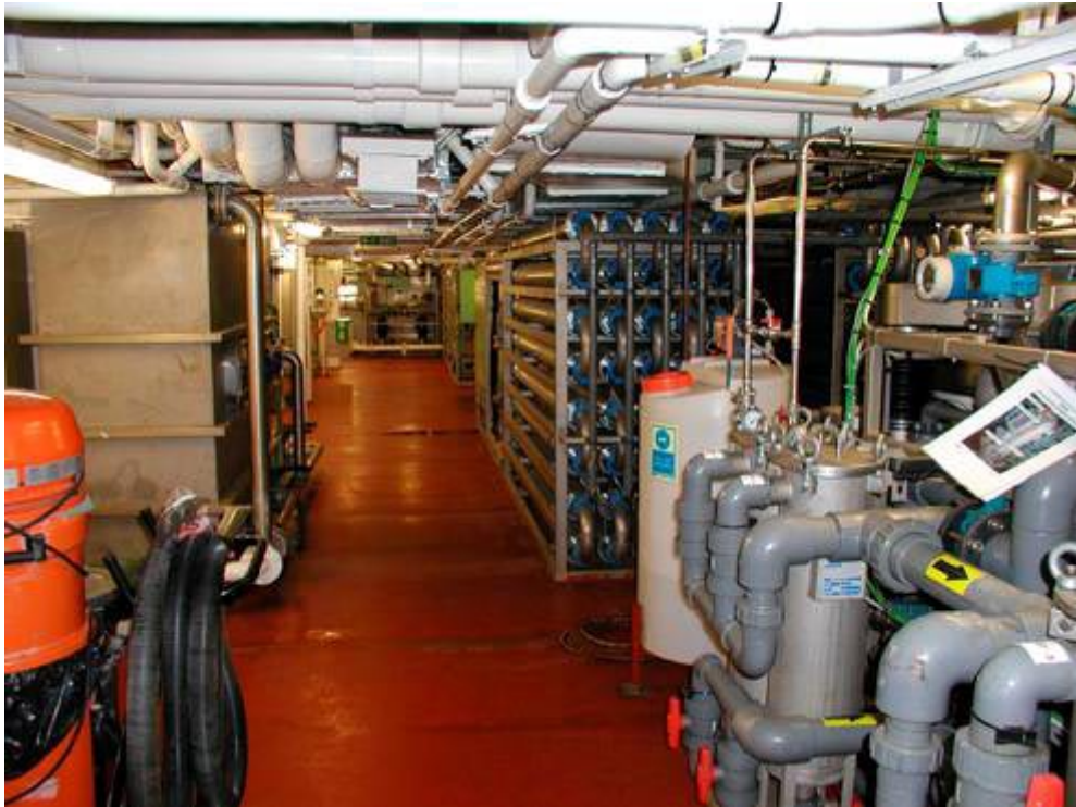
ROCHEM LPRO Systems Installed on Holland America Line Vista Class Vessels
