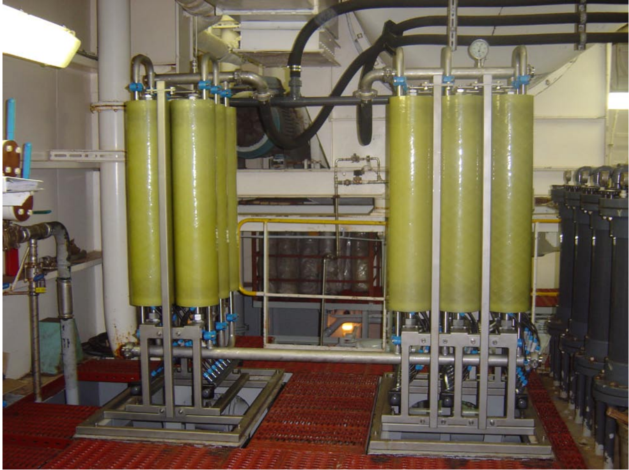
ROCHEM High Pressure Reverse Osmosis Modules Installed on Carnival Vessel
