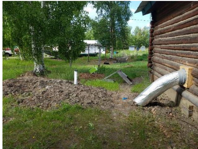
Seepage Pit, Chalkyitsik
