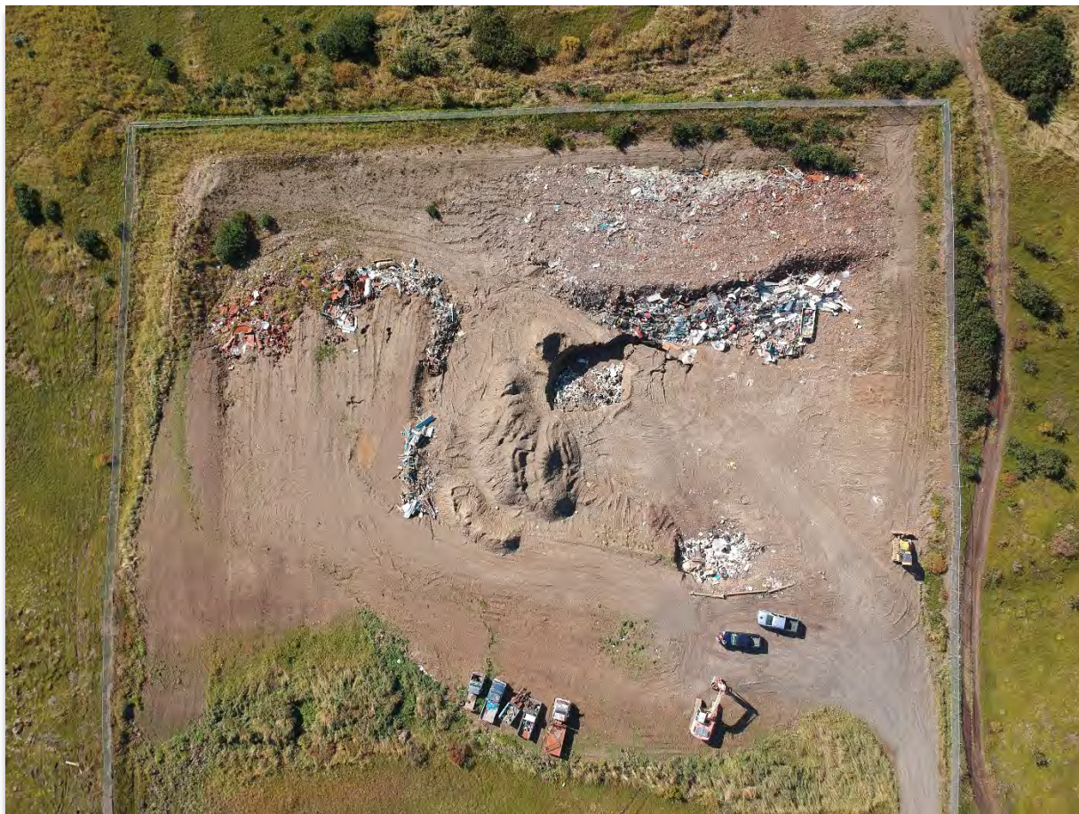
Area fill landfill with two separate working faces demonstrating excellent consolidation. The household garbage working face is near where the cars are parked, allowing easy drop off by the public. The larger working face towards the back of the landfill is for metals.
