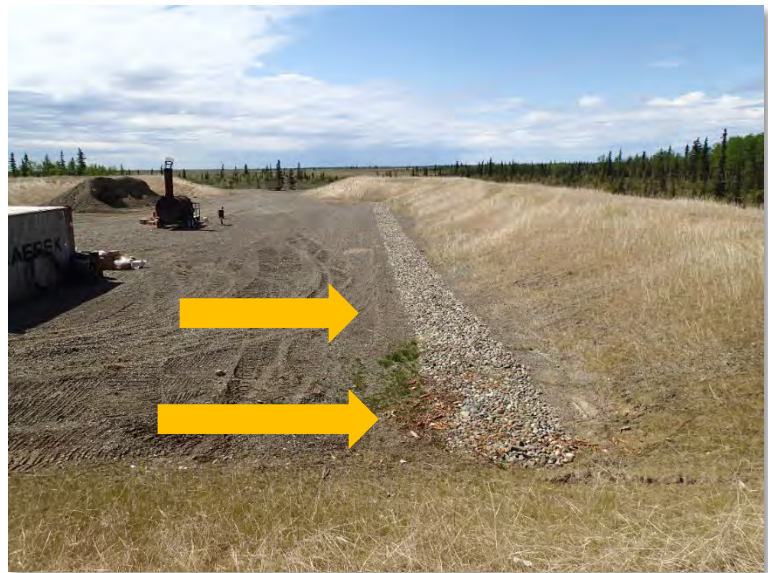
Engineered drainage system to prevent storm water from coming into contact with the waste.
