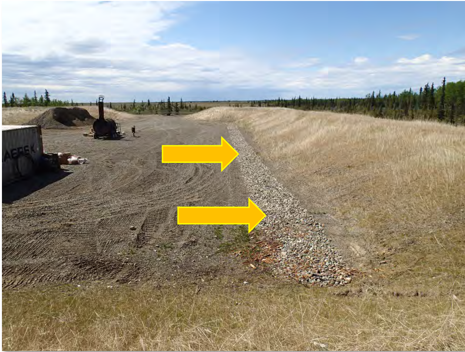
Engineered drainage system to prevent water from running onto the waste from the berms surrounding the facility.
