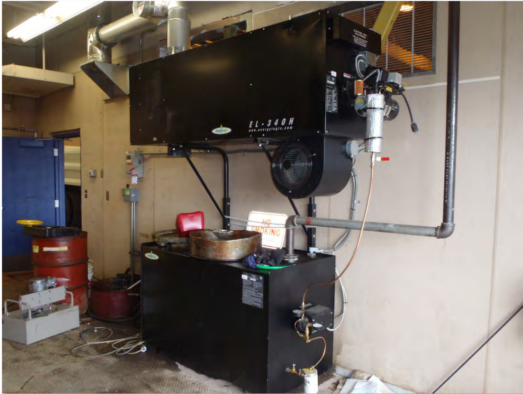
EPA approved used oil burner for energy recovery to heat community building.
