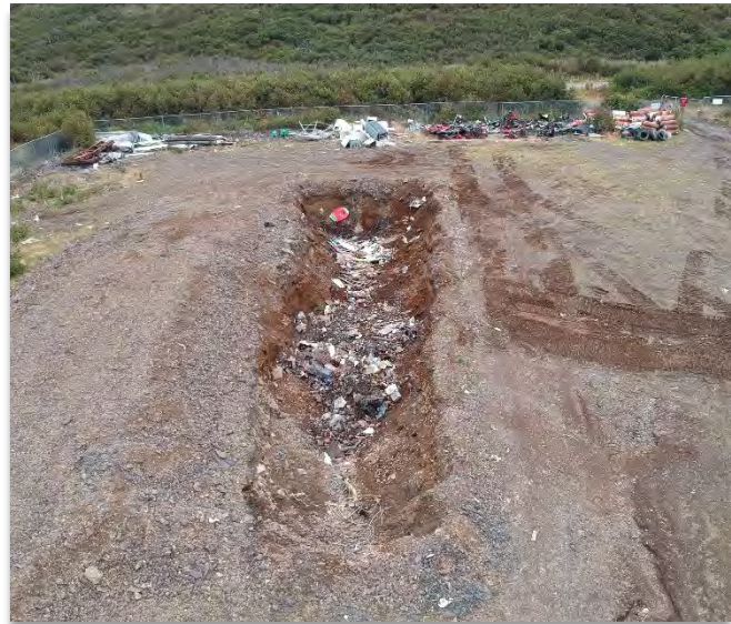
Trench-and-Fill landfill. All the waste is consolidated into one half of the trench. Notice that the waste is not spread across the site.
