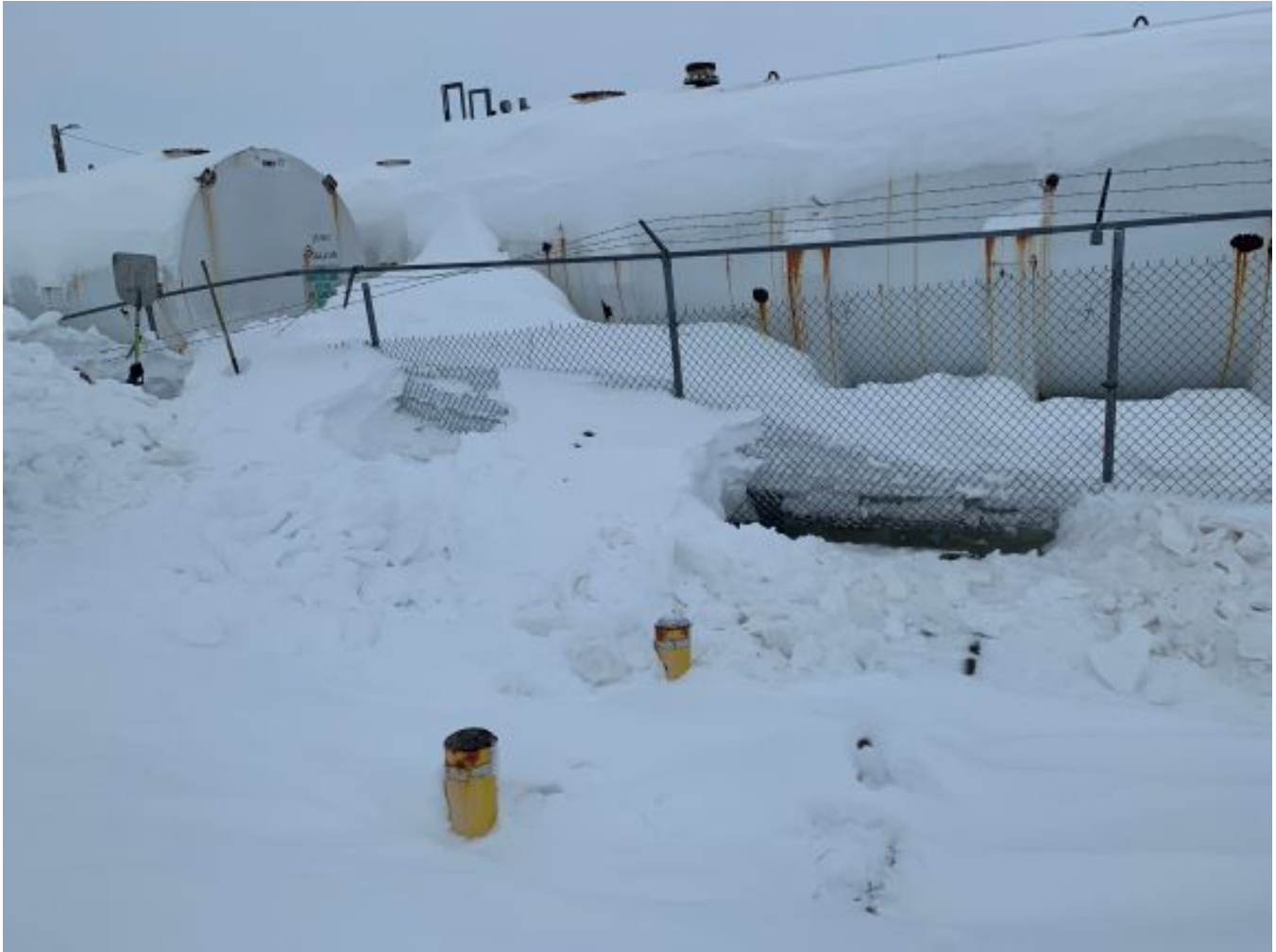
Tank farm where spill was found outside of secondary containment area. (Photo provided by Scott Stiker, March 3, 2021)
