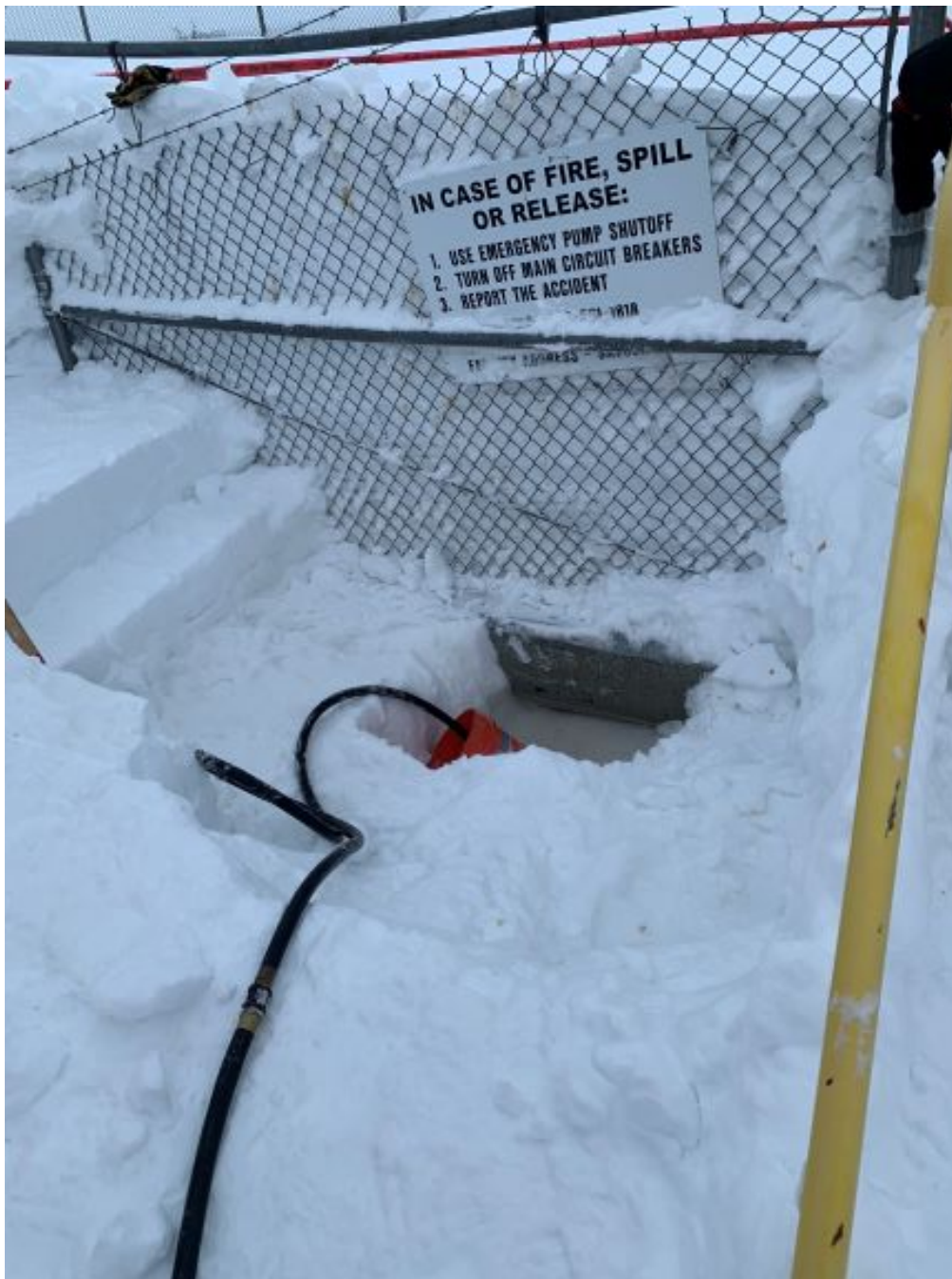
The suction end of pump recovering product from an excavated hole in the snow drifts at a low point within the secondary containment. (Photo provided by Scott Stiker, March 1, 2021)
