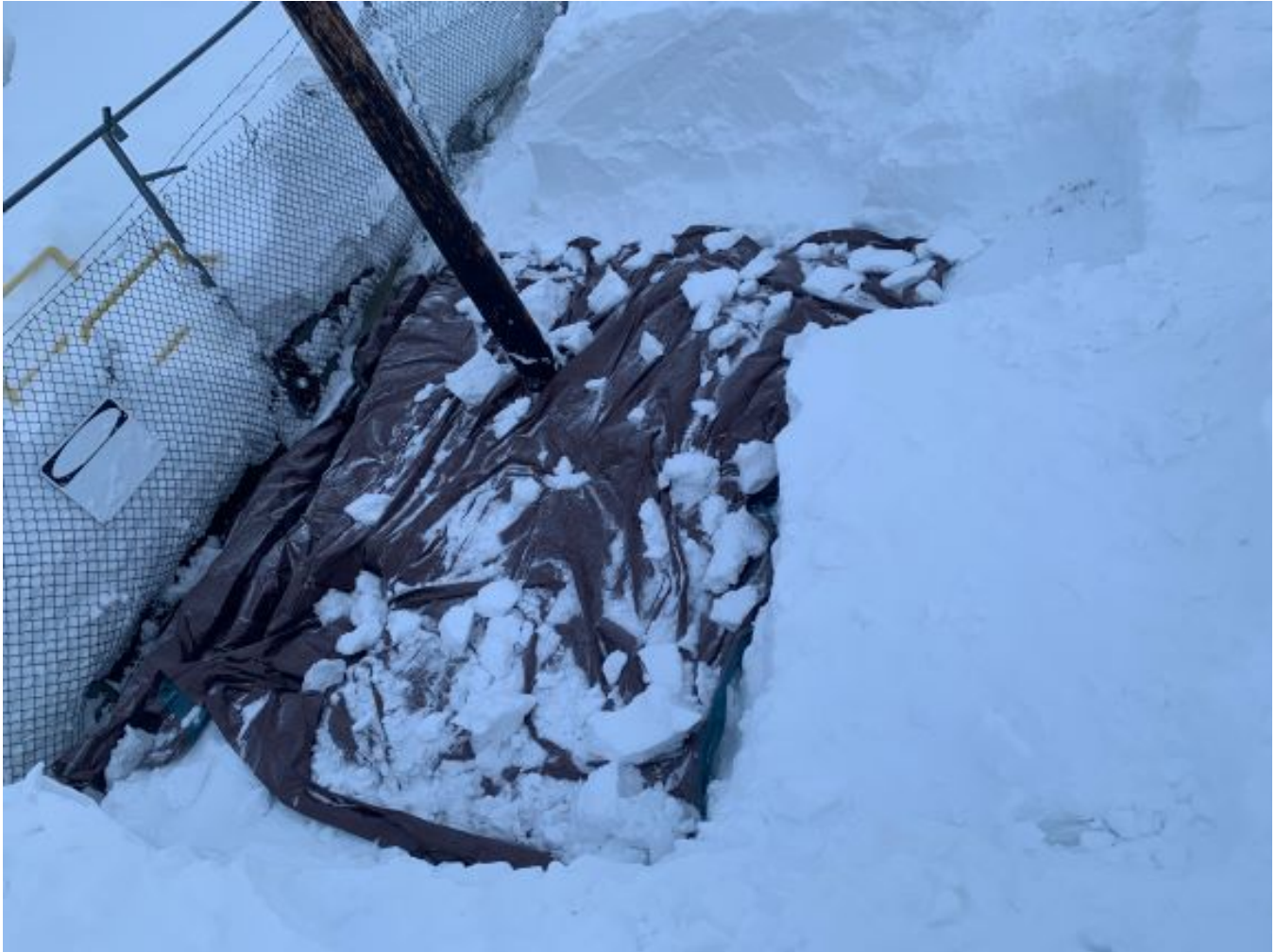
Photo 2. Excavation site where diesel was found outside of secondary containment. The area was covered in preparation for high winds and snow. (Photo provided by Scott Stiker, March 3, 2021)
