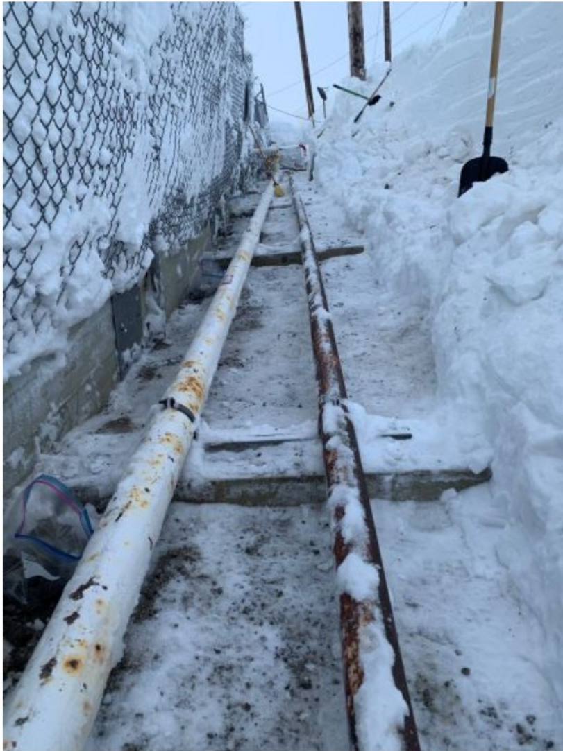
Photo 1. Snow removal on the west wall outside of secondary containment of the tank farm to check for additional contamination. (Photo provided by Scott Stiker, March 24, 2021)
