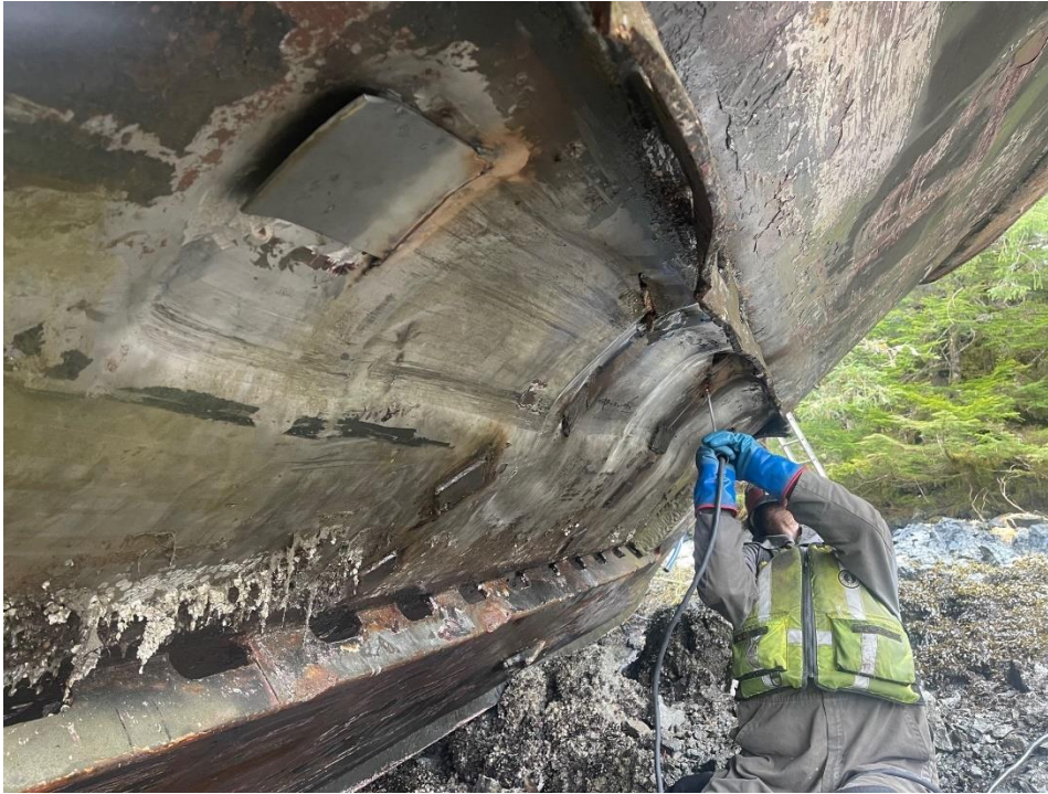
Figure 3. Global Diving and Salvage, Inc. crewmember continues fabrication welding on the hull of the Western Mariner on March 25 th . Photo by Global Diving and Salvage, Inc.
