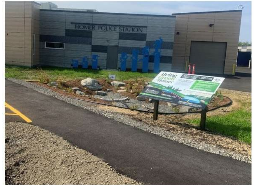
New RAIN GARDEN - site drainage directed to garden to slow peak storm water and filter sediments
