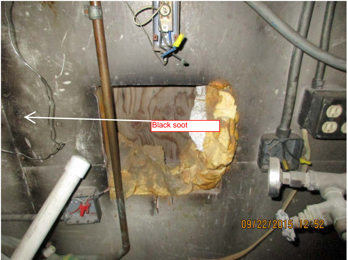
Figure 3 – Black soot on wall in Tank room.
