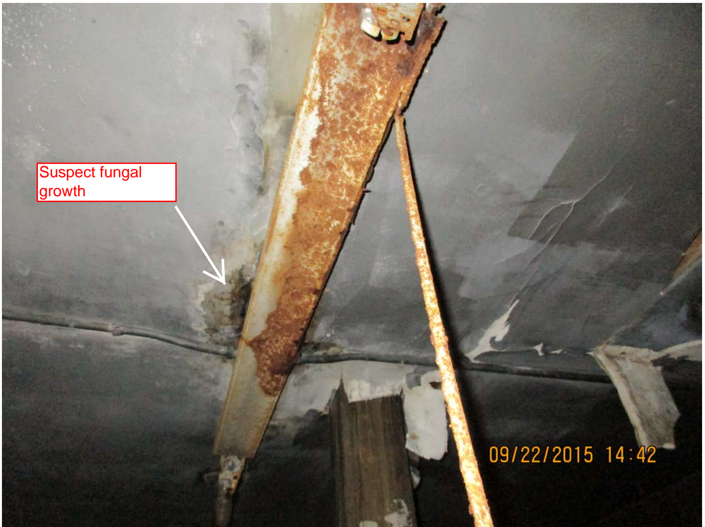
Figure 7 – Suspect fungal growth on gypsum wall board ceiling of the mechanical room.
