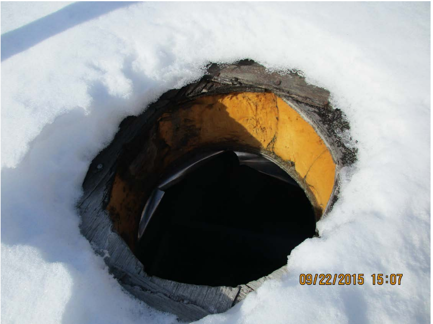
Figure 9 – Missing roof flashing directly above the mechanical room.
