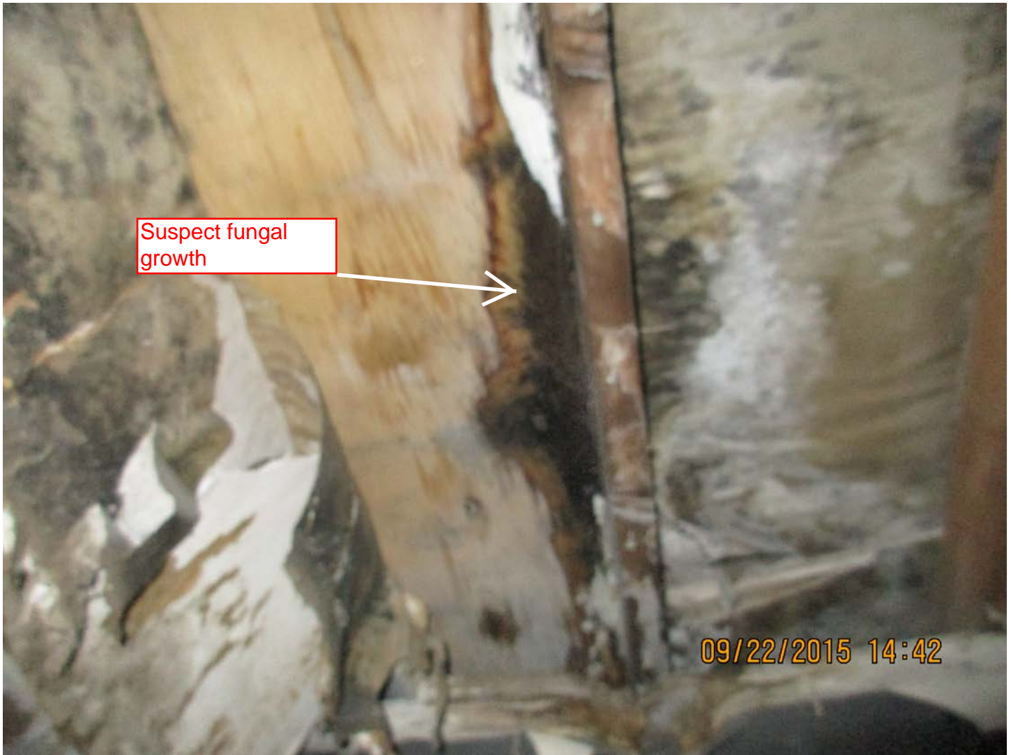
Figure 6 – Suspect fungal growth on wood members in the ceiling of the mechanical room.
