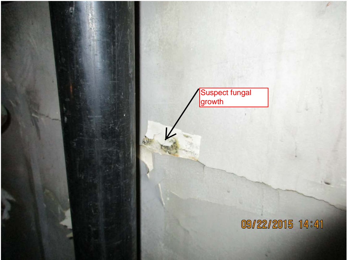
Figure 5 – Suspect fungal growth between the paint layer and gypsum wall board in the mechanical room.
