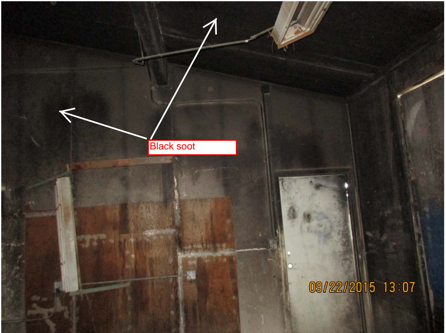
Figure 4 – Black soot on walls and ceiling of shop area S1.
