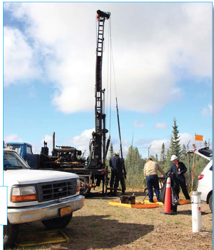
(Right) A Flint Hills contractor drills into the ground to install a new monitoring well, one of 80 installed this summer. (FHRA photo)
