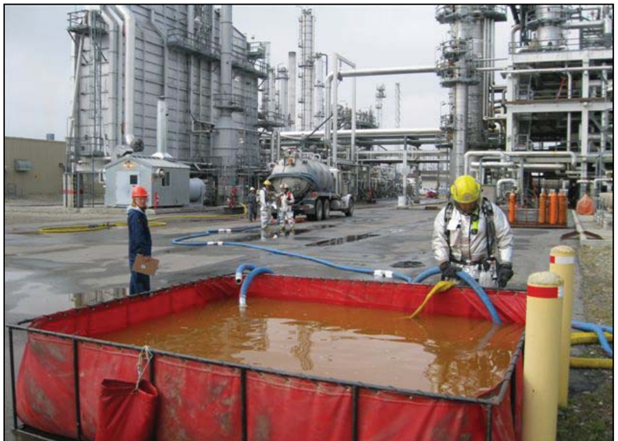
Ann Farris, DEC’s project manager, is shown inspecting pumping operations. (DEC photo)
