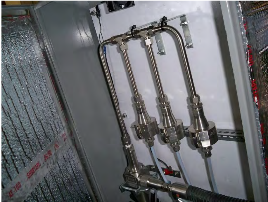
Figure 3-4 Temperature Controlled Filter Sampling Cabinet
