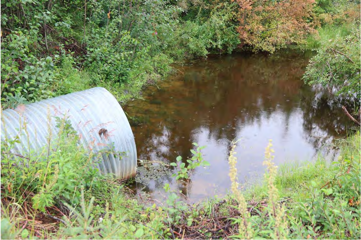
Perched Culvert at PRM Area 3
