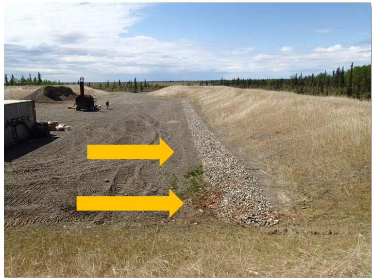
Engineered drainage system to prevent storm water from coming into contact with the waste.
