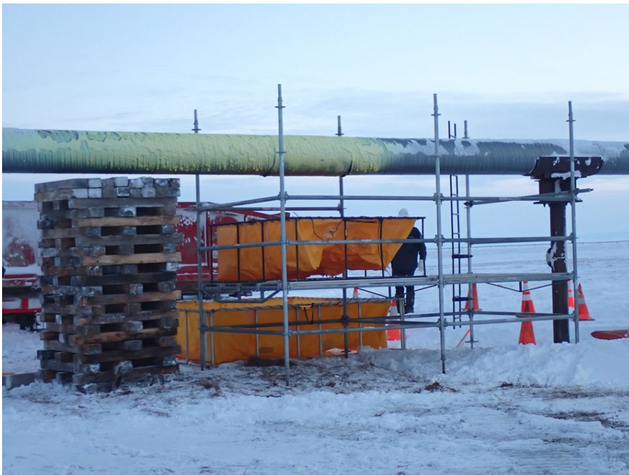
Figure 4. Working on getting scaffolding for pipeline jacket inspection. Fold-a-tank placed under pipeline in case of residual condensate on January 17, 2023. Photo provided by Alaska Department of Environmental Conservation.
