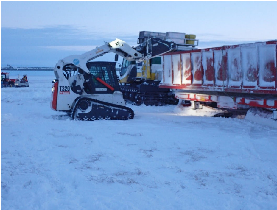
Figure 5. Loading contaminated snow into a bin for transport to Deadhorse on January 17, 2023. Photo provided by Alaska Department of Environmental Conservation.
