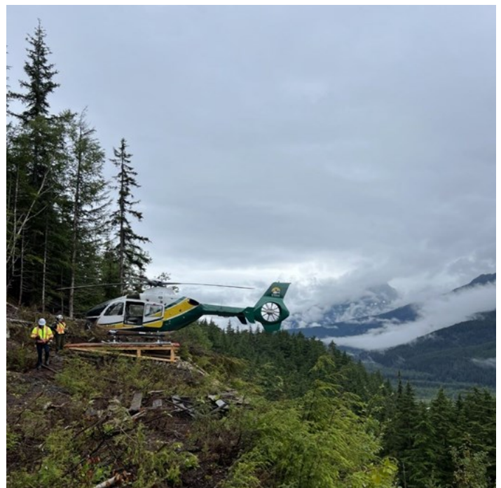
Temporary helicopter landing pad at the 5900 portal of the Tulsequah Chief Mine Site, 2024.
