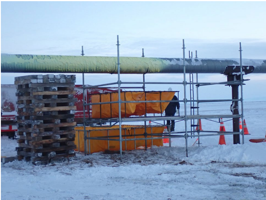
Figure 4. Working on getting scaffolding for pipeline jacket inspection. Fold-a-tank placed under pipeline in case of residual condensate on January 17, 2024. Photo provided by Alaska Department of Environmental Conservation.
