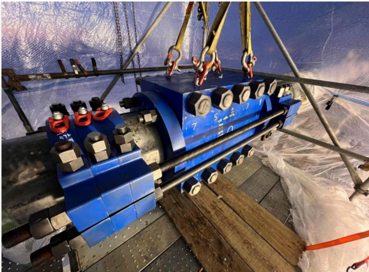
Figure 6. Repair Clamp installed on affected section of pipeline on January 28, 2024. Photo provided by Harvest Alaska, LLC.
