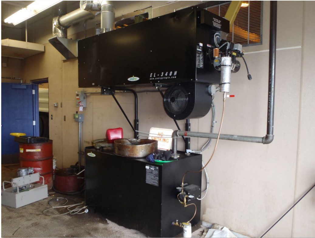
EPA approved used oil burner for energy recovery to heat community building.
