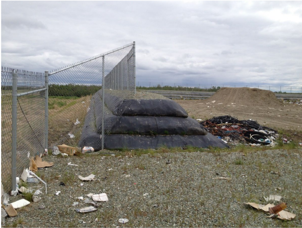
Berms and fencing surrounding an above-grade area fill in wetlands. The berms provide a wall against which to compact waste and help keep the landfill separate from the wetlands, while the fencing helps to contain windblown litter.
