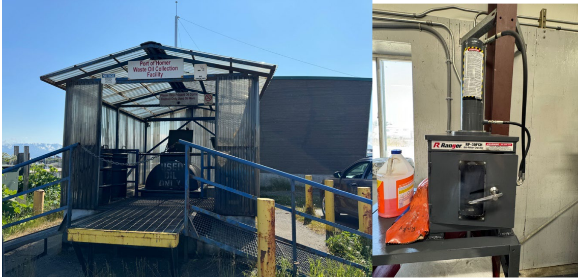
Figure 15: Homer uses an extensive waste oil collection network which is then used to heat their workshop with a burner. Their facility also boasts an oil filter crusher (right) to maximize reuse.
