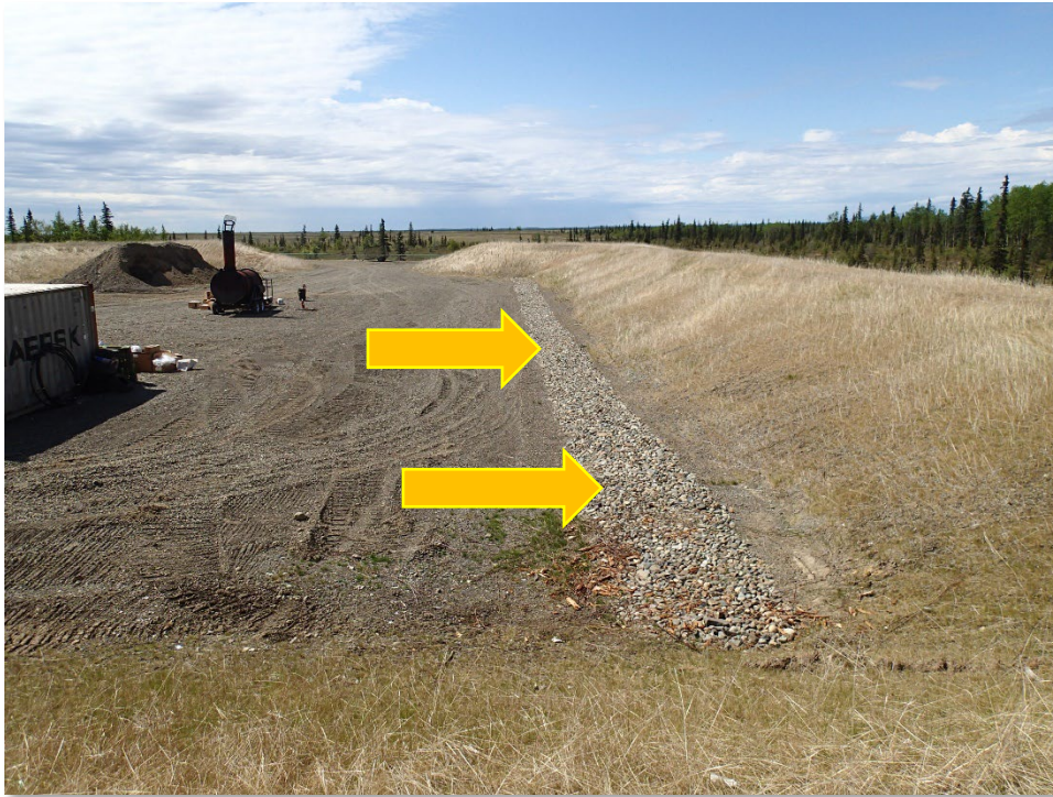
Engineered drainage system to prevent water from running onto the waste from the berms surrounding the facility.
