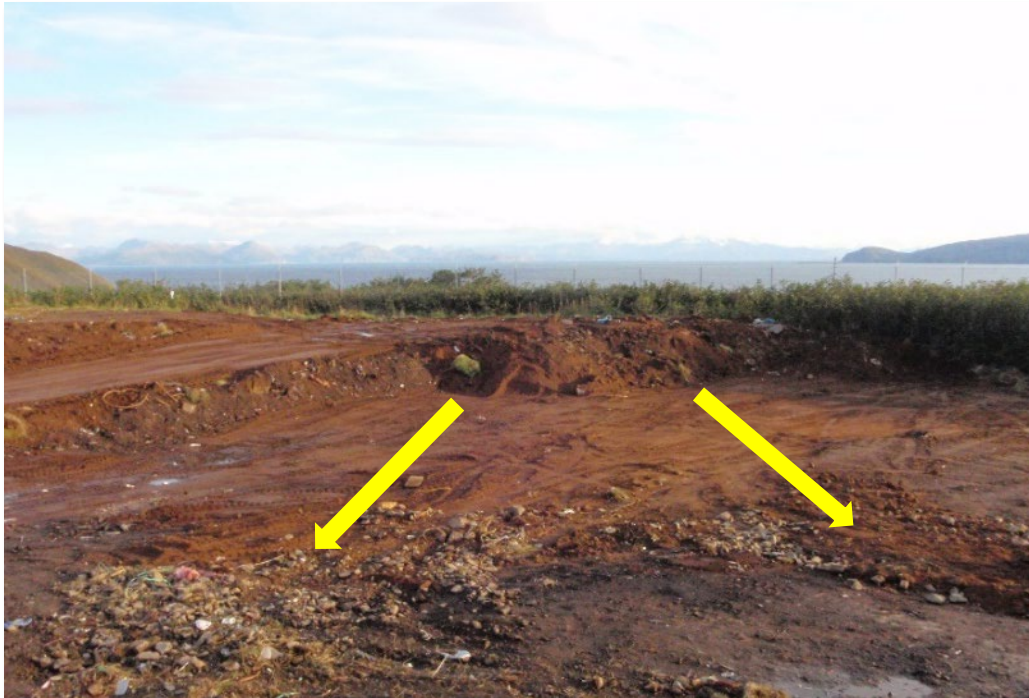
Cover material at the working face graded to promote water drainage away from the waste. Water is draining away from the working face following the arrows.
