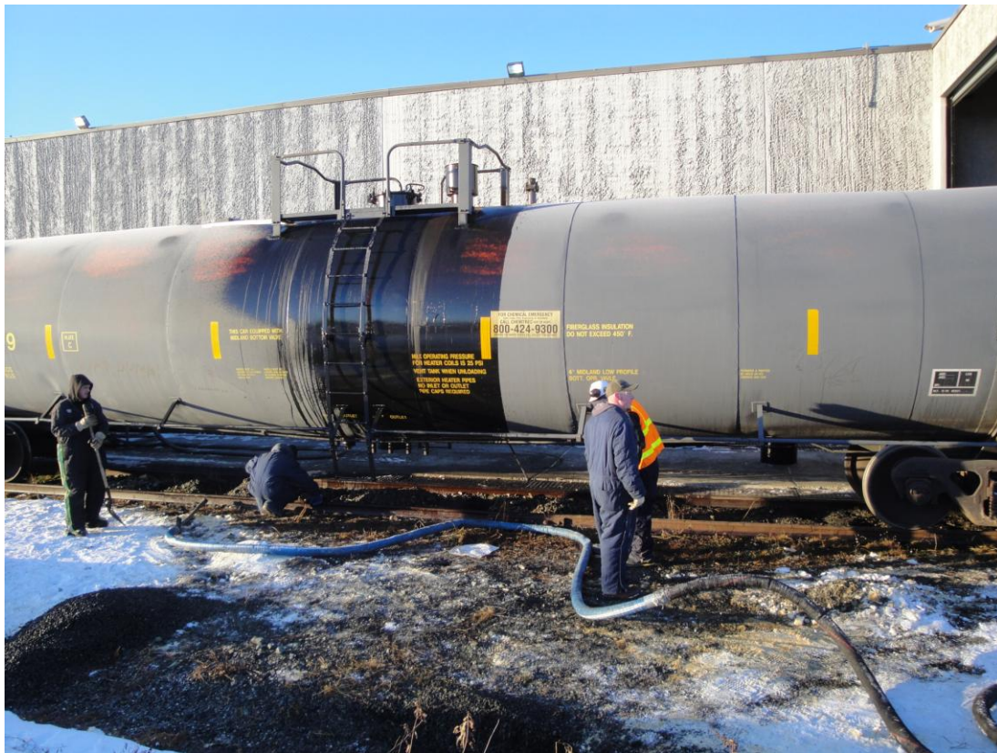
Univar corrosion inhibitor spill recovery efforts, November 16, 2010. Photo by ADEC.
