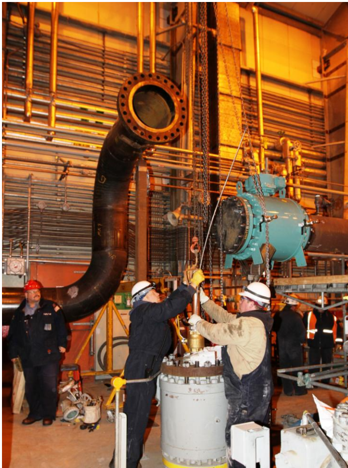
Workers installing the bypass pipeline inside the metering building. This new line will bypass existing pipe, where a leak was discovered on January 8, and reroute the crude oil flow to a new access point into the booster pump building. (1/15/11)
