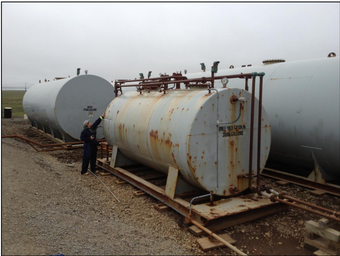
July 19, 2012: Wes Ghormley (ADEC) inspecting day tank which overflow caused the incident
