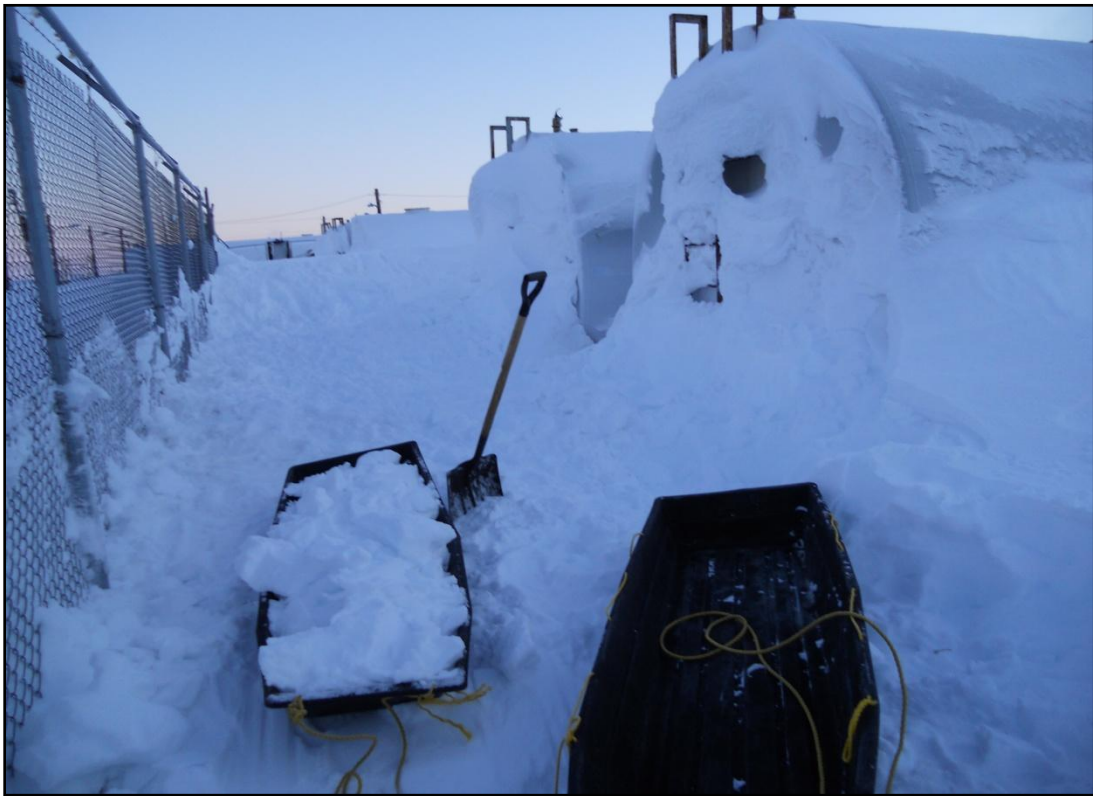
January, 2012: Response equipment used to remove uncontaminated snow from the tank farm
