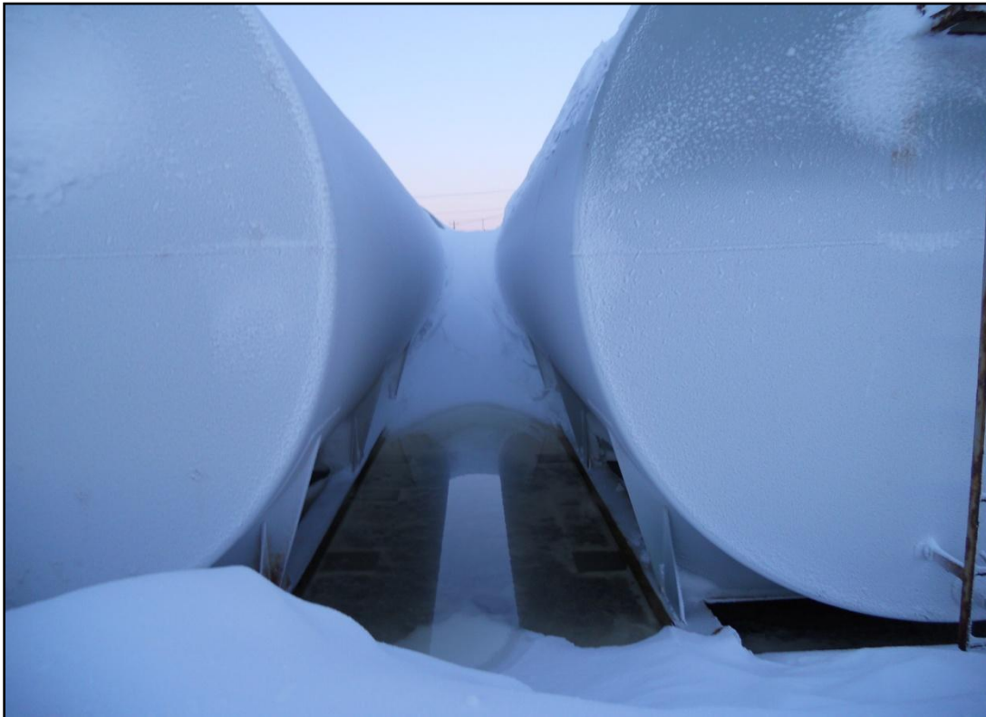
January, 2012: Pooled diesel fuel within the tank farm
