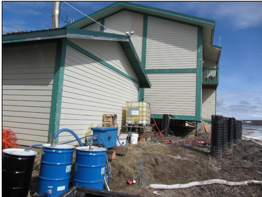
Spill area with recovery sumps and water treatment system (RSE photo)
