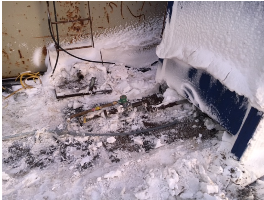
Photo showing the broken fuel line between the 5,000 gallon tank and pump house, January 9, 2017. (Photo/NSB)
